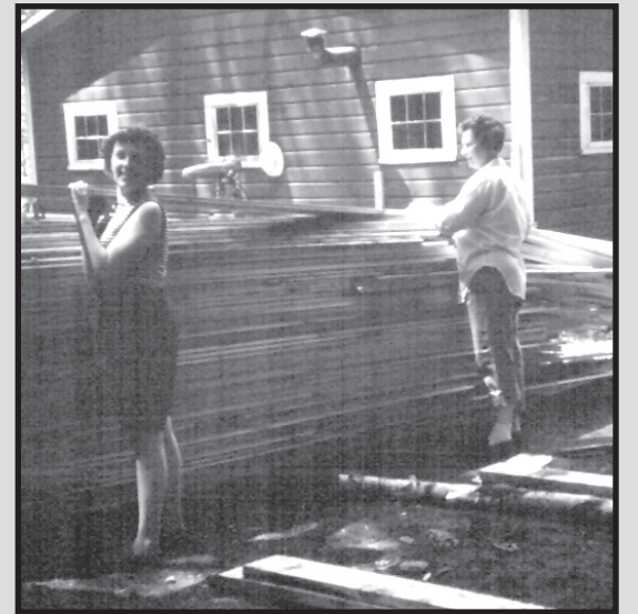
Betty Jane (left) and Marion help carry lumber during the construction of Camp Berger in Winchester Center.
